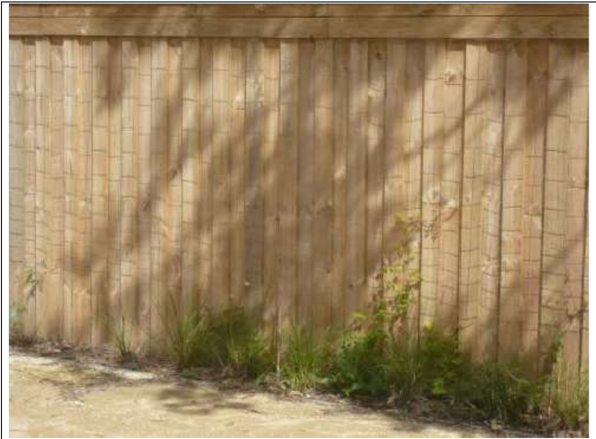
Figure 6.5 – Boundary Acoustic Fence at Monitoring Locations 1 & 2
