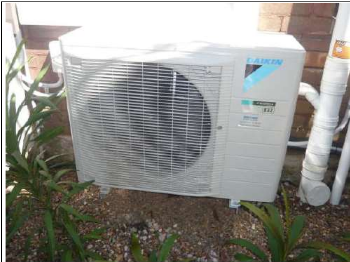
Figure 6.14 – AC Condenser Unit (3)
