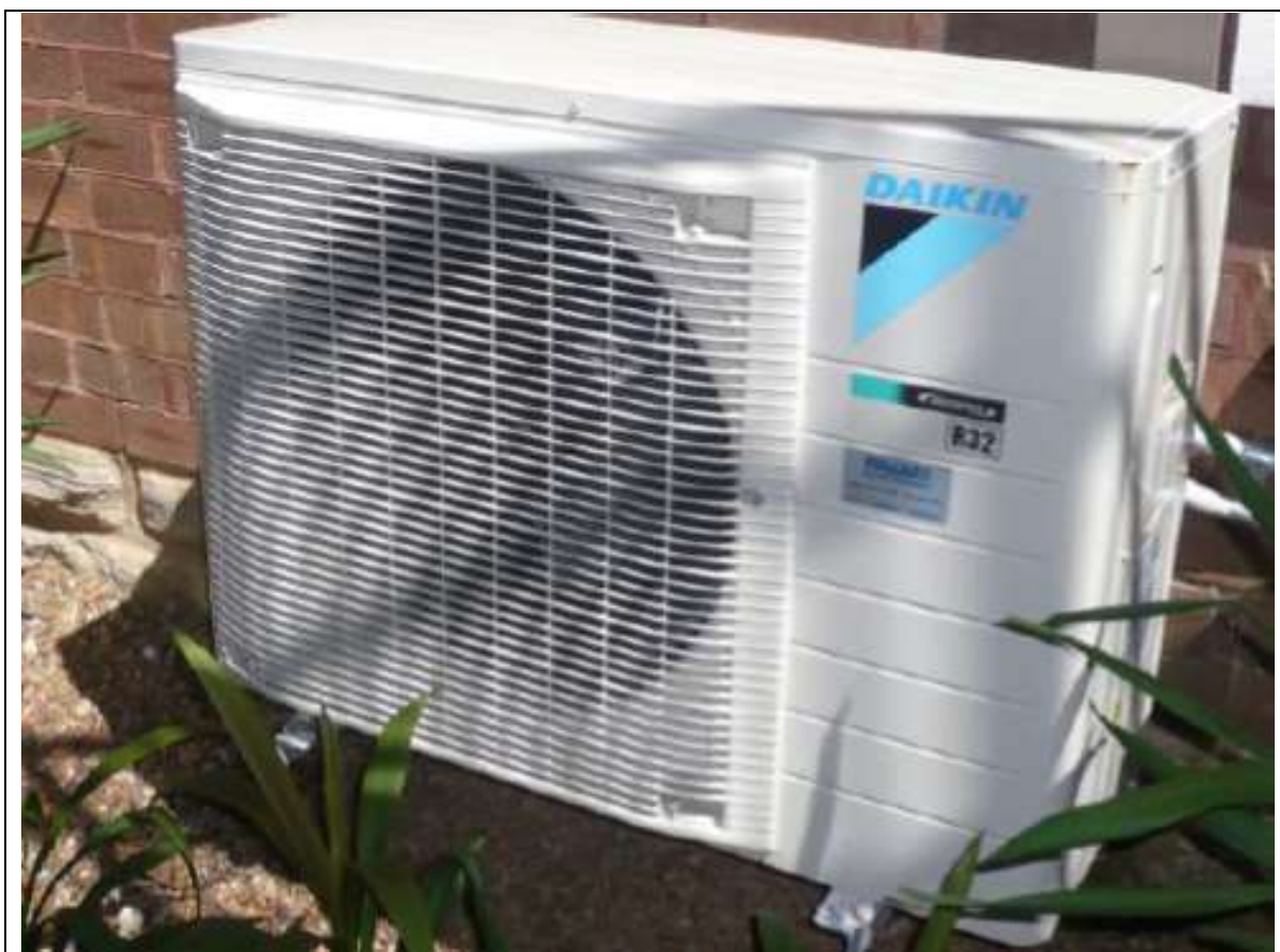
Figure 6.15 – AC Condenser Unit (4)
