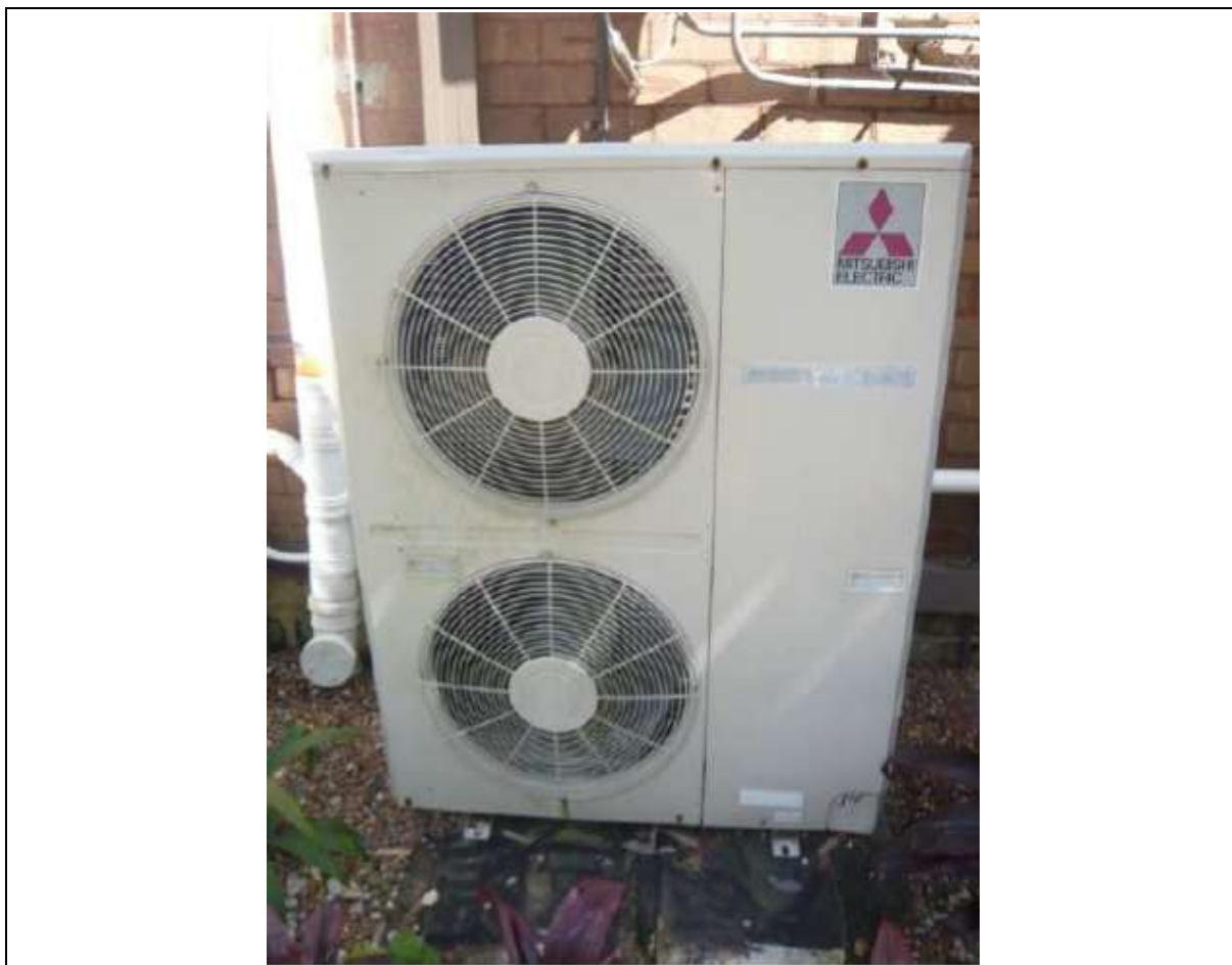
Figure 6.13 – AC Condenser Units (2)
