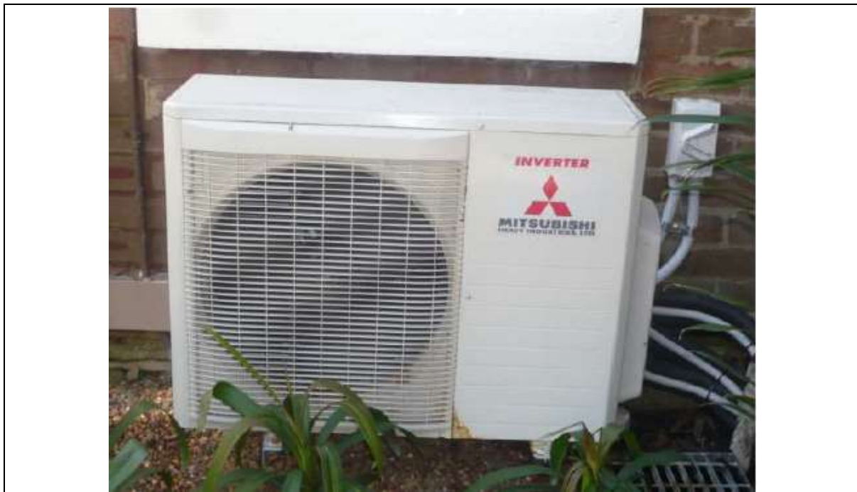
Figure 6.12 – AC Condenser Unit (1)
